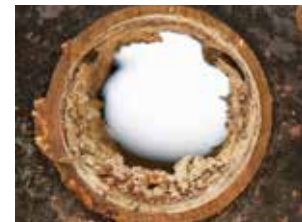
Unprotected tankless: Failed at 5.8 years of operation and 136,000 gallons
